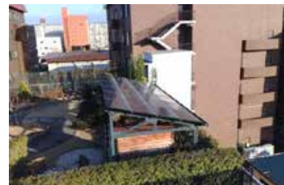
大学5号館屋上(3kwh)
